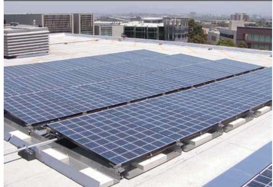
Roof top systems
